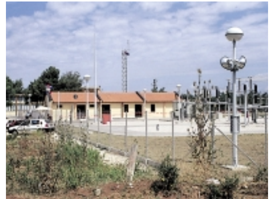
TS Katoro 110/35/10(20) kV Katoro
