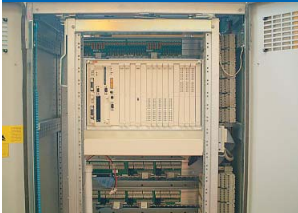
Nova procesna stanica agregata
