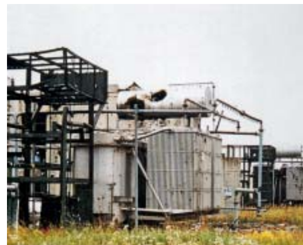
Energetski transformator 400/110 kV
