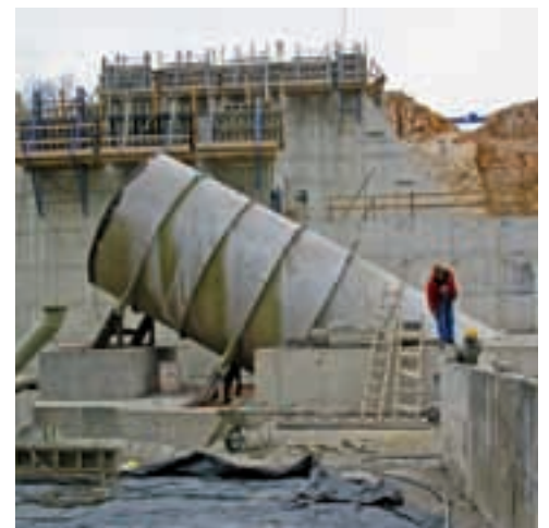
Cjevovod agregata B
