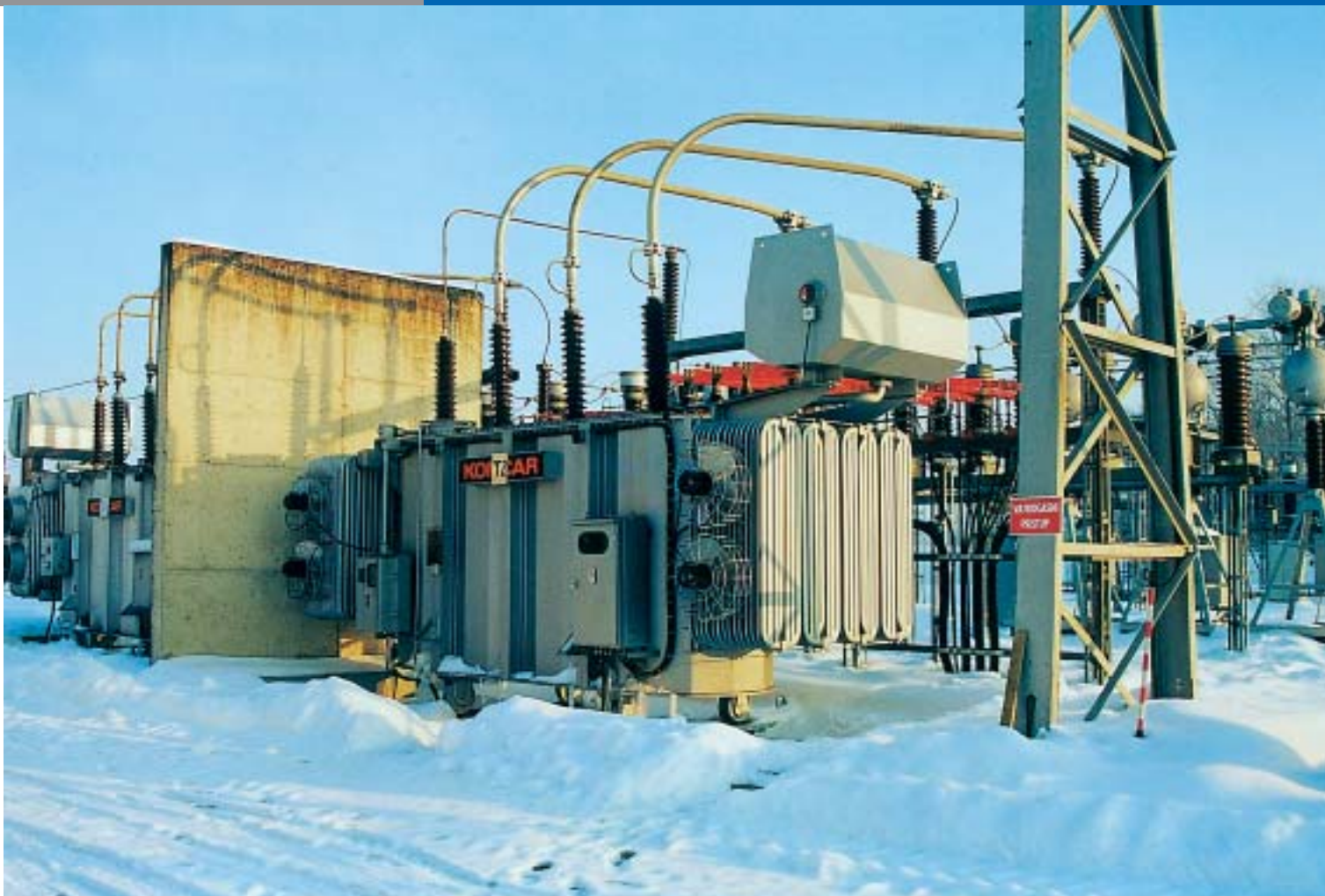
110 kV polje (novog 110/20 kV) transformatora 2 TS Zdenčina
