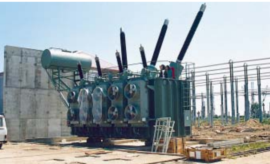
Energetski transformator 400 kV - 1...
